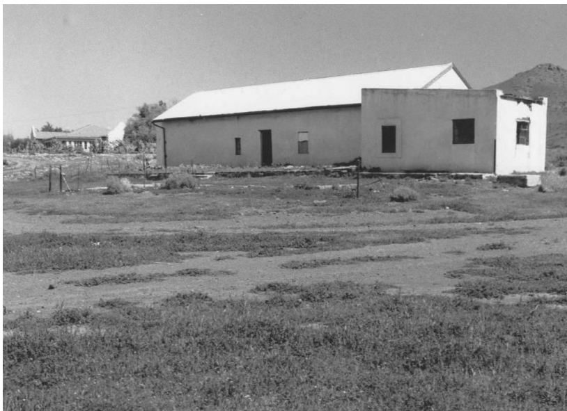
Figure 6. After the disastrous fire of 1949, leading to the collapse of the gable, the house was given a corrugated iron roof. The fourth house can be seen in the background to the left. (AP 1999)
