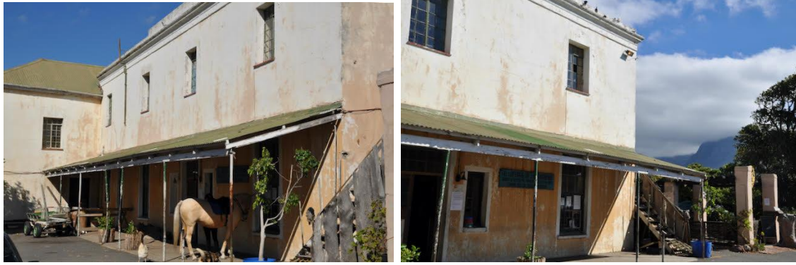
The main historic building in 2012, since partially collapsed.
